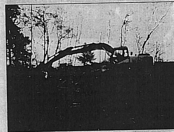
SUBMITTED PHOTO Crews have been using earth moving vehicles to clear foliage along the highway near Chinook.
