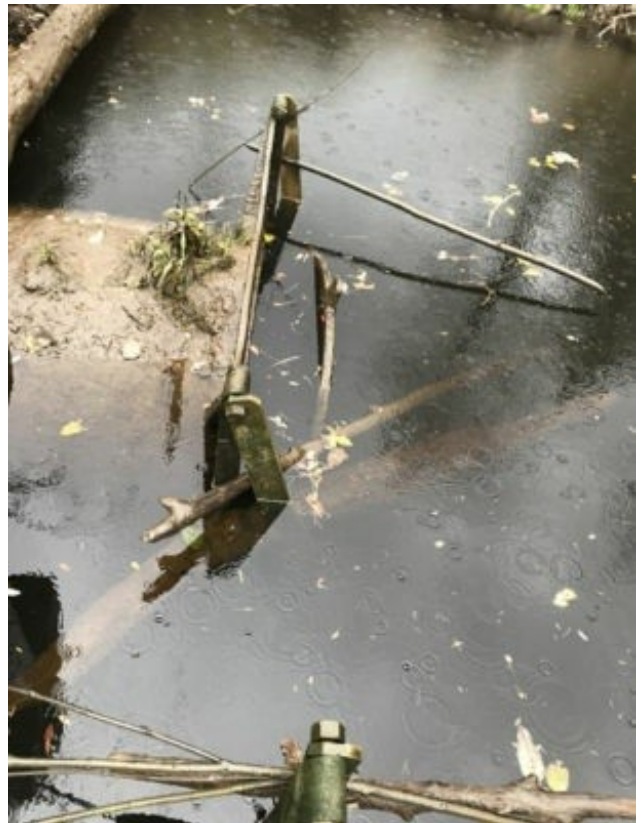
Resource extraction: Repairing failing infrastructure can be costly, complicated and controversial. Courtesy of CREST
