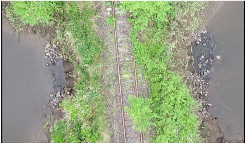
Photo captured from above the existing culverts that will be removed and replaced with the dual span 60' bridge.
