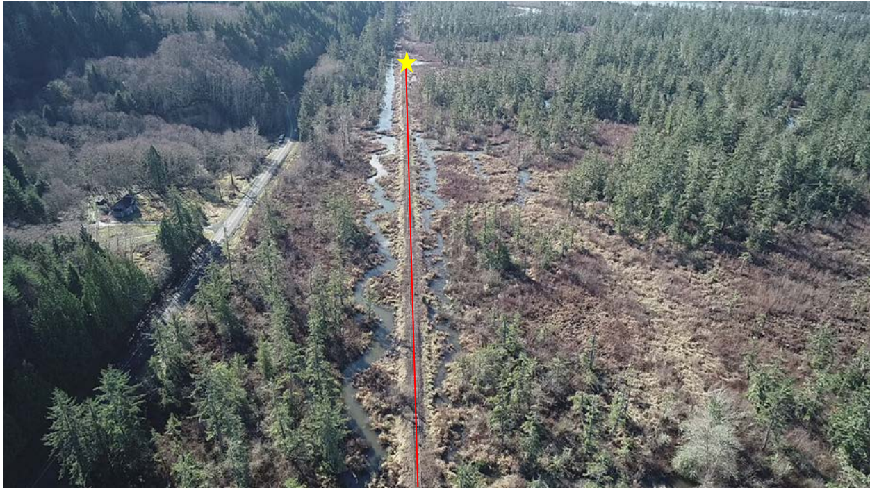
Photo captured from the eastern side of project area, looking to the west. Red line indicates access route along existing railroad, yellow star indicates the location of the culvert removal and installation of the 60' double span bridge..
