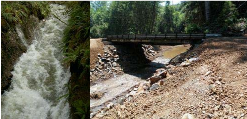
Big Creek velocity barrier (left); new bridges on the historic meander (right).
